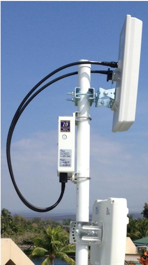
Qbridge and sector antenna installed at ocean-front resort
